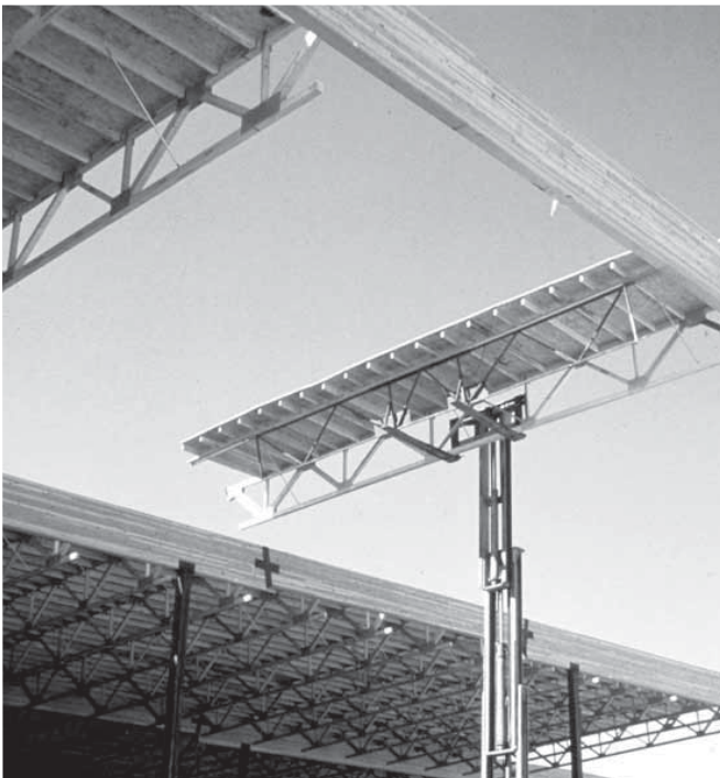
Erecting glulam structures is often much faster and more cost effective than comparable steel systems because there is no need for specialized trades.
